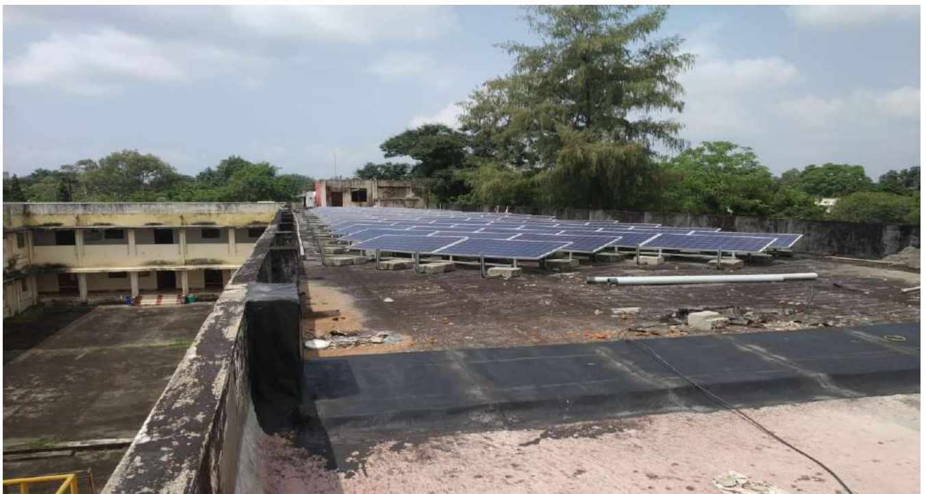
Figure 9 : Solar panels installed on roof
